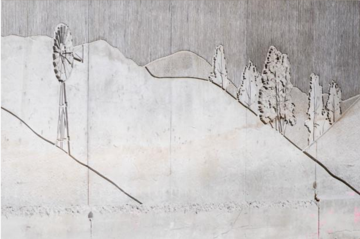
Cement engravings are pictured along the retaining wall of the 60 freeway Lemon Avenue westbound on ramp at the Caltrans construction site in Diamond Bar on Wednesday, February 7, 2018. (Photo by Raul Romero Jr, Contributing Photographer)
