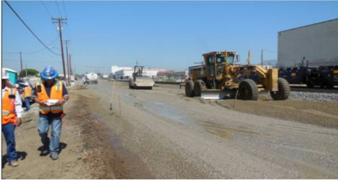
Work is underway on the Baldwin Avenue Grade Separation Project in El Monte. Photo Credit: ACE
